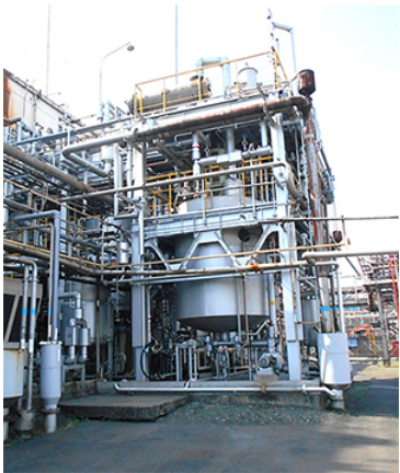
Distillation Recovery Facility
