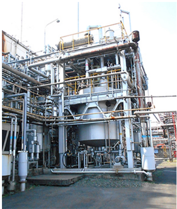
Distillation Recovery Facility
