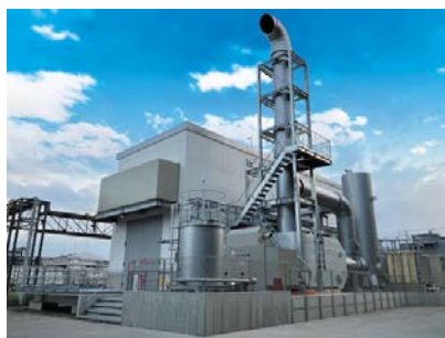
Exterior View of the newly-installed Gas Co-generation System
