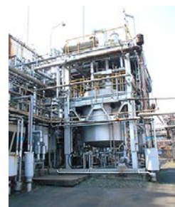
Distillation Recovery Facility
