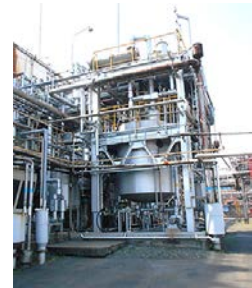
Distillation Recovery Facility
