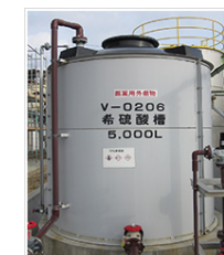
We make sure that workers recognize the hazards of the chemical substances to which they could be exposed.
