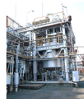
Distillation Recovery Facility
