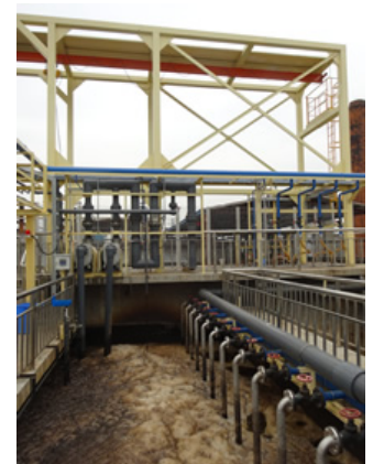
Wuxi Advanced Kayaku Chemical's wastewater treatment facility
