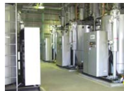
High-efficiency once-through boilers
