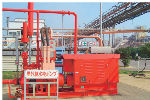
Fire Protection Equipment Fukuyama Plant
