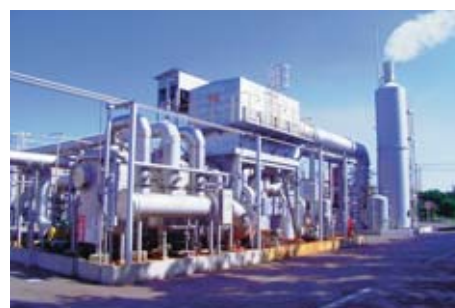
Exhaust gas decomposition equipment
